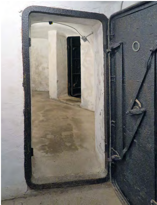
Gas-proof blast door in Mussolini's original shelter. Some of the rubber seal was still in situ. Space was very limited and certainly not large enough for many beyond the immediate family
